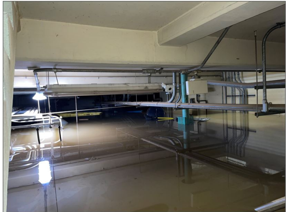
GBPS During Hurricane Ida Sept-2021 Two (2) Lower Levels Under Water
